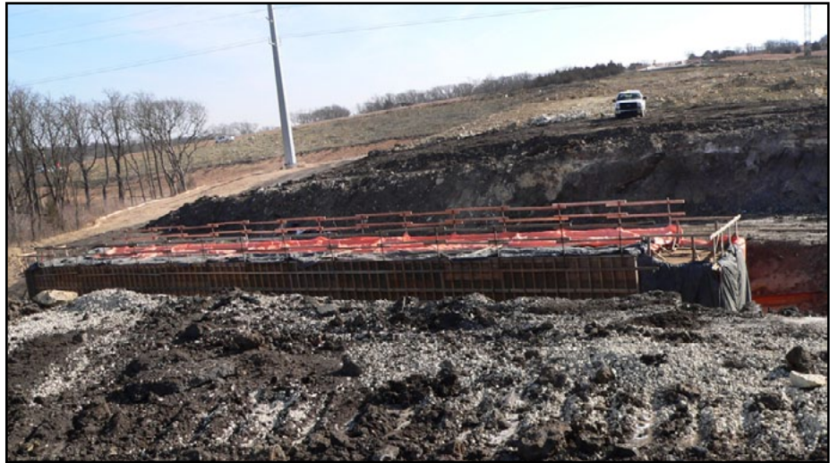
Above is an eastbound view of a K-18 box culvert where concrete was recently placed. Below is a westbound view of the remaining K-18 work to be finished.
