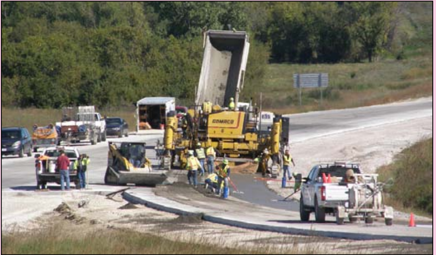
Work on the U.S. 169 pavement reconstruction in Allen County continues with concrete paving on the Minnesota Road exit ramp. Emery Sapp & Sons, Inc., of Kansas City, Mo., is contractor on the seven-mile project between Delaware and Minnesota roads. The cost of construction is $16.1 million. Aaron Frits' road squad and Mark Hurt's bridge squad designed the project.
