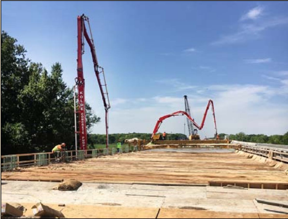
For the Allen Creek bridge on the Kansas Turnpike near MM 130 on I-335/KTA, crews pour the new deck.
