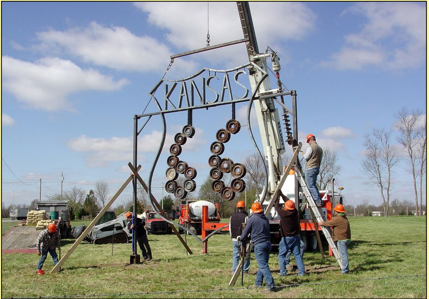
KDOT crews from Columbus, Pittsburg and Chanute install a metal Kansas 66 shield near the roundabout at U.S. 400 and K-66. Members of the Riverton High School FFA constructed the shield, which now enhances sections of historic Route 66 in Kansas.
