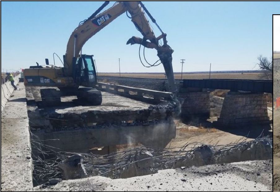
Demolition of the second bridge in Hamilton County is currently taking place.
