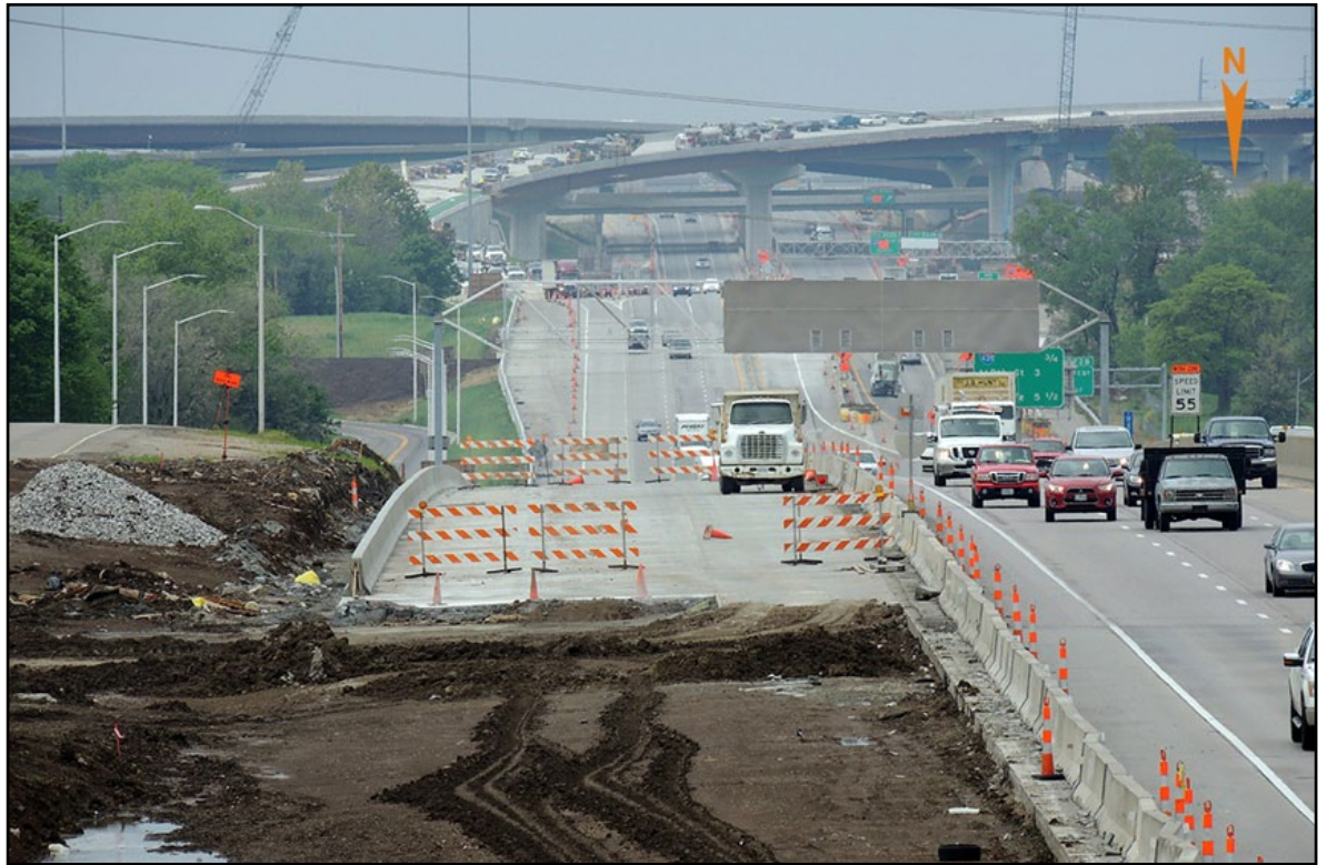
The Johnson County Gateway project included reconstruction and capacity improvements within the I-435, I-35 and K-10 interchange area along with improvements at several major local interchanges.
