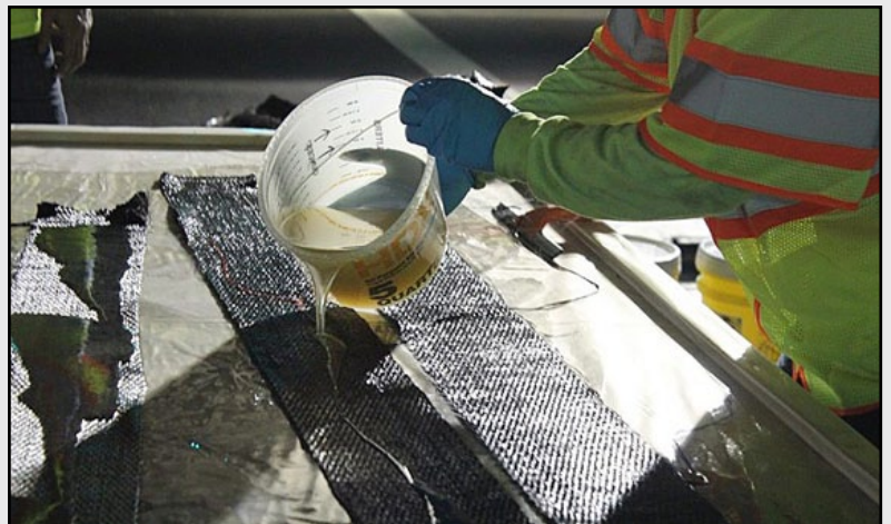
Carbon fiber strips were used to fix girders on two bridges in Arizona.
