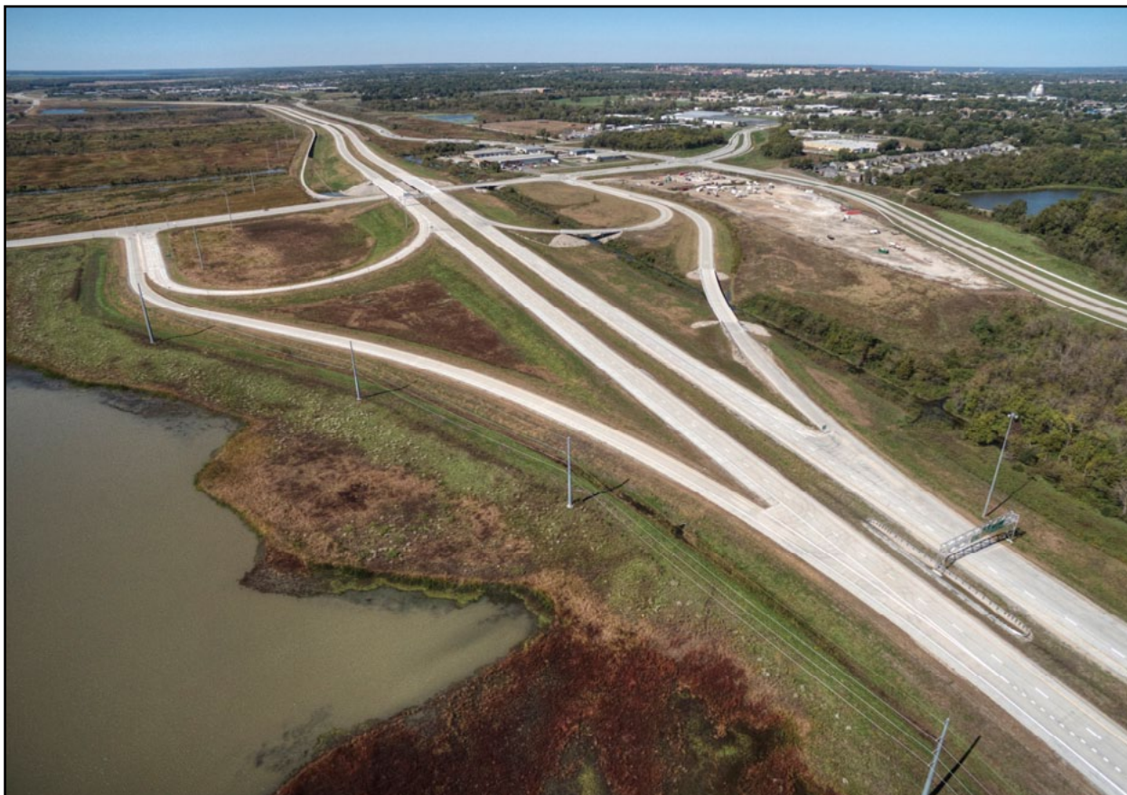
Construction work on the South Lawrence Trafficway East Leg included 24 bridges, 29.4 highway lane miles, 16.3 miles of local roads and three new interchanges.
