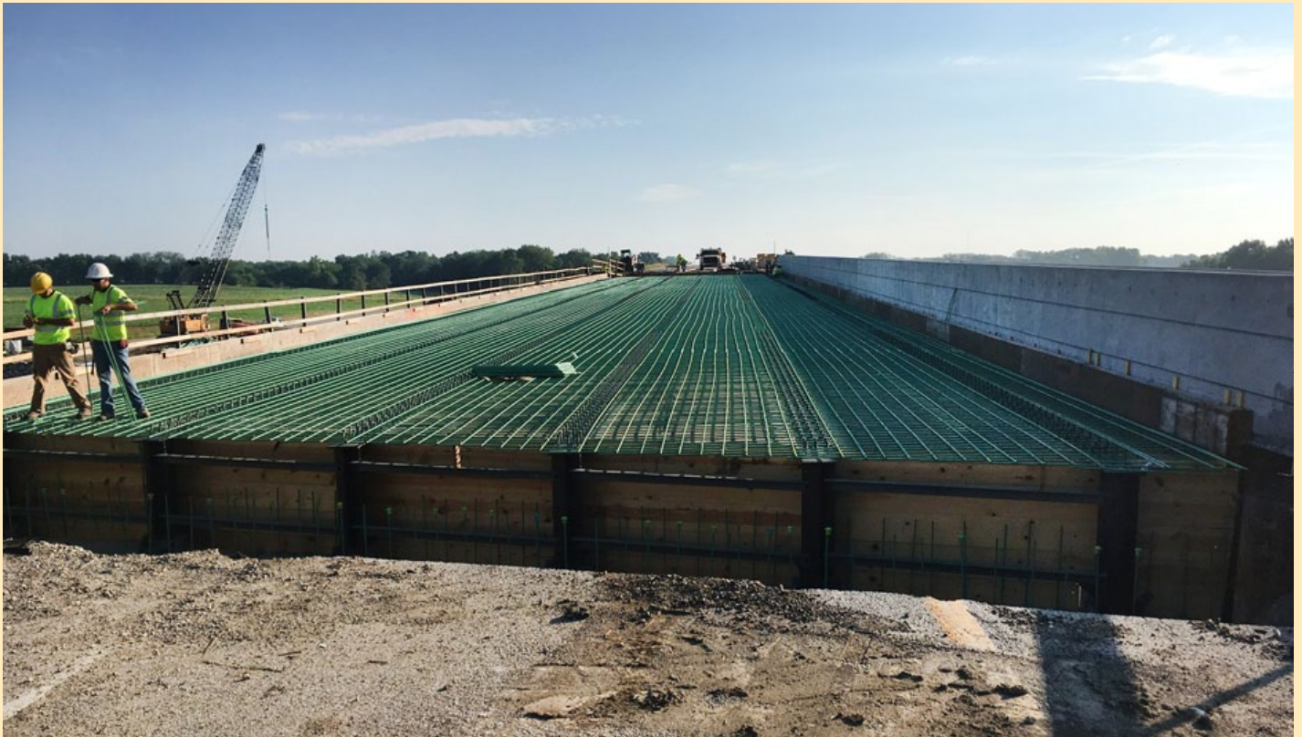
A two-year project to reconstruct two bridges over Dagoon Creek and remove two bridges crossing an abandoned railroad track in Osage County is underway about 20 miles south of Topeka. The northbound bridge was reconstructed in 2016 and work on the remaining bridges will occur in 2017.
