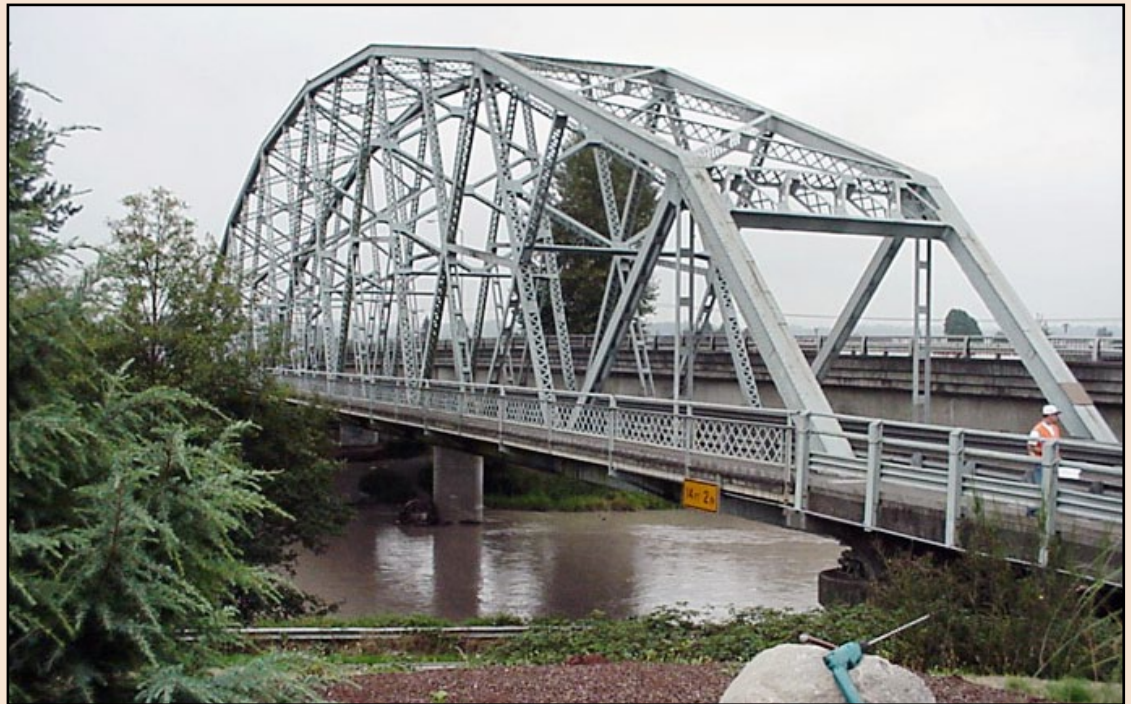
The Washington State DOT is looking for a new home for this bridge built in 1925.
