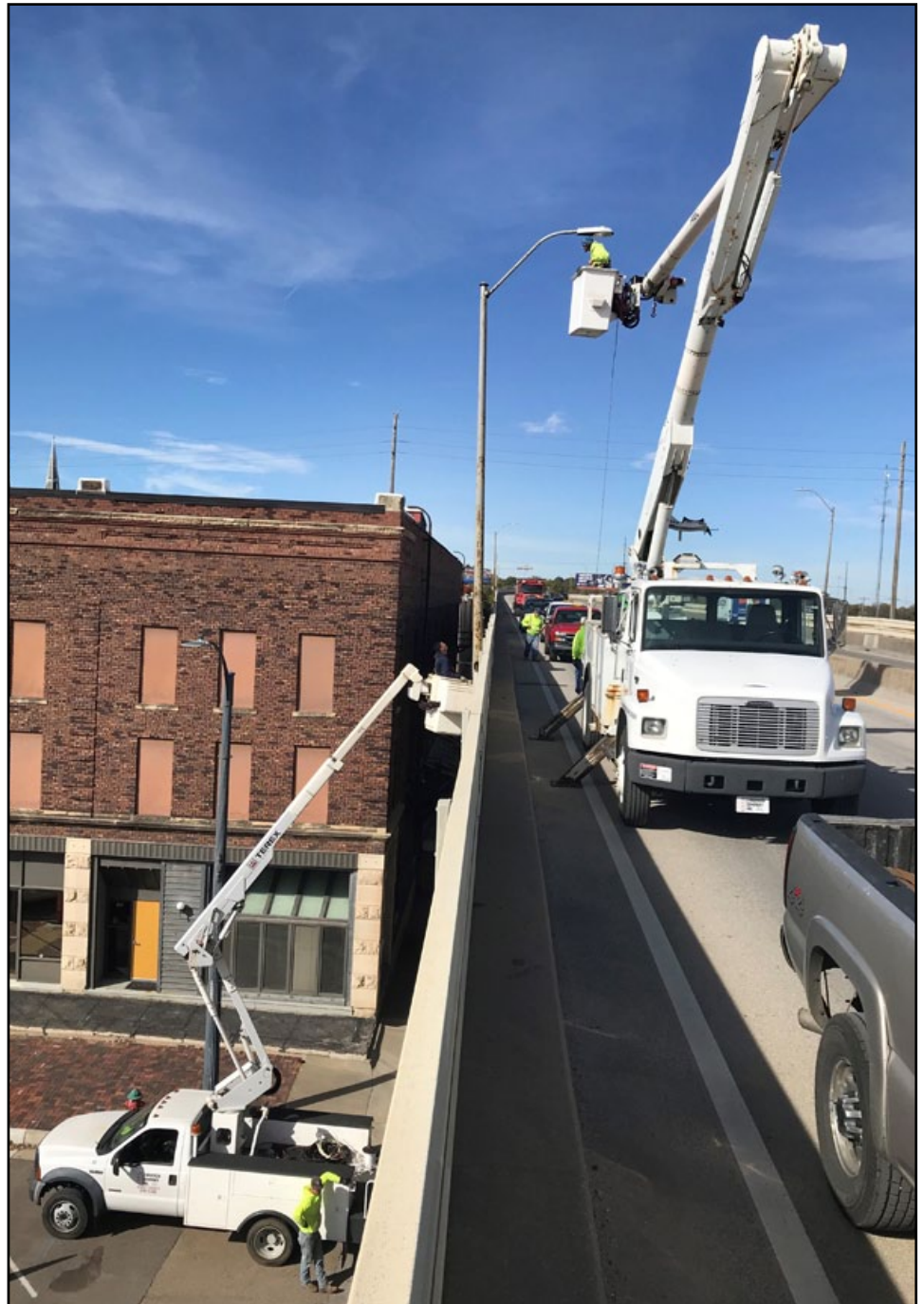
New LED fixtures are installed to increase visibility as part of a lighting improvement project along the Polk-Quincy Viaduct in Topeka. J Warren Company Inc. of Topeka is the contractor on the $159,000 project that took place in October.
