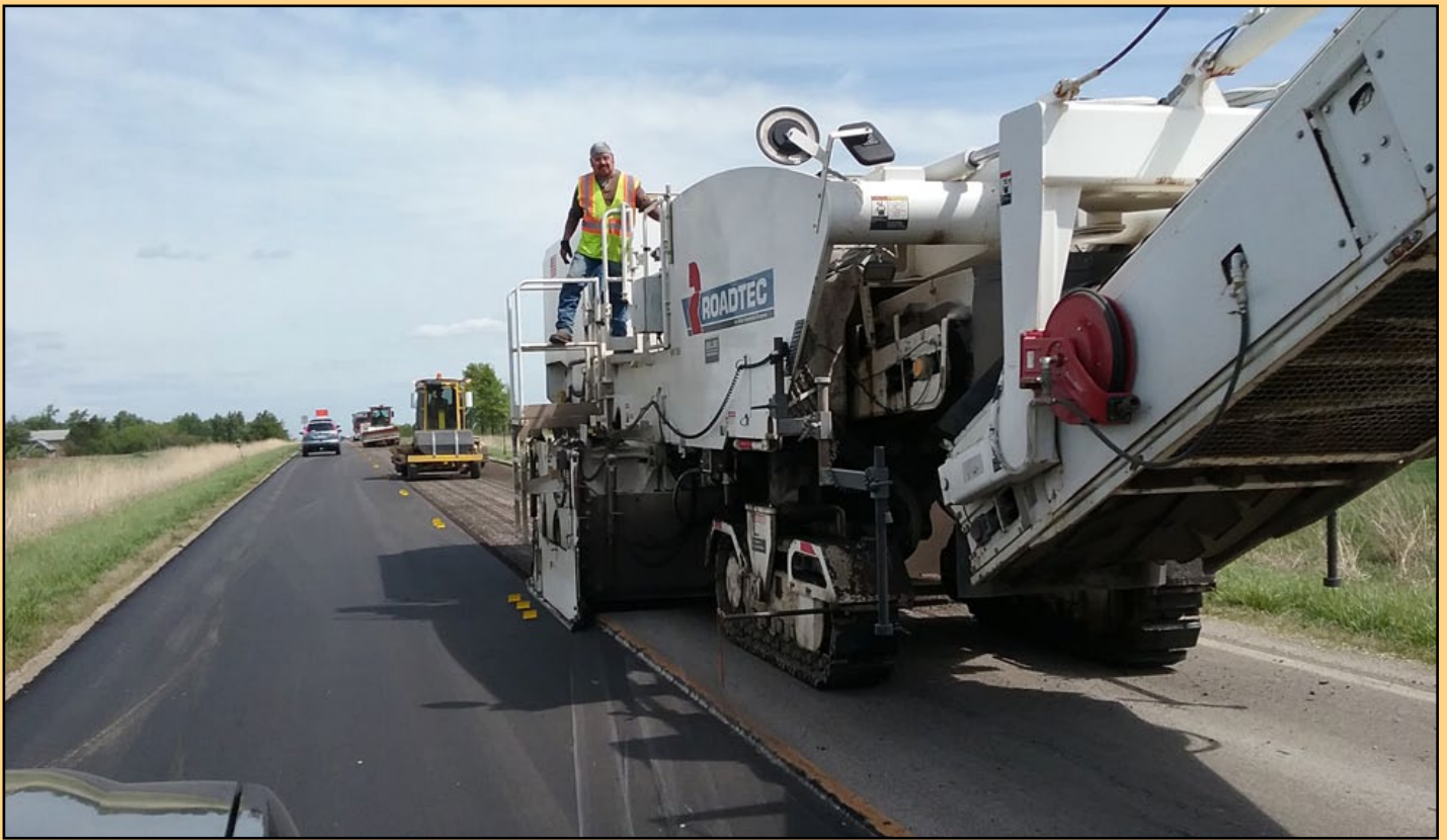
K-31 is being resurfaced with a mill and asphalt overlay from U.S. 59 at Garnett northwest to I-35 (above). Shilling Construction of Manhattan is contractor on the 30-mile project.
