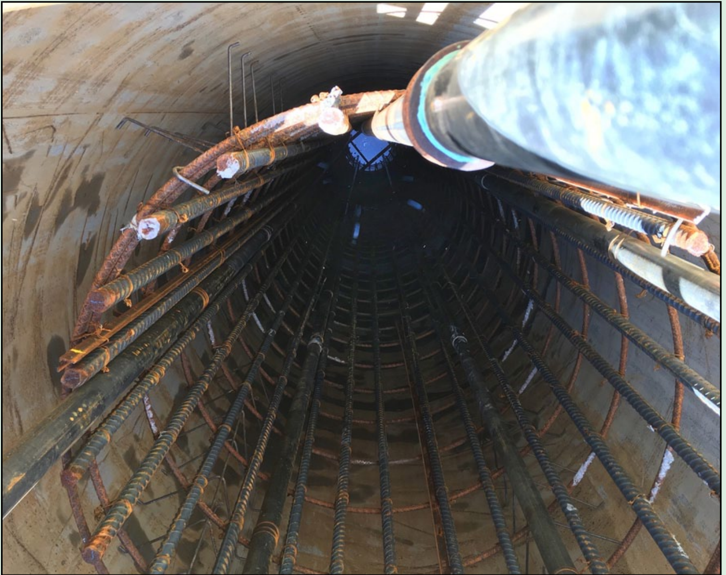
Crews pour concrete in the drilled shafts at the Osage County bridge project, located at mile marker 157 on I-335/KTA.
