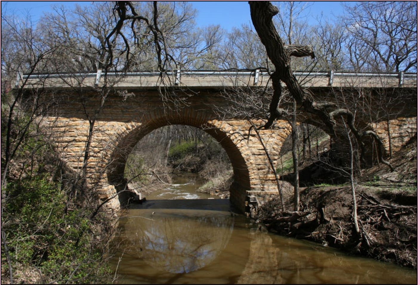
KDOT employee Neil Croxton photographed the stone arch bridge on K-181 north of Sylvan Grove in Lincoln County. This bridge was built in 1903. KDOT built a new bridge just to the west of this structure in 1994 and the stone bridge is now used for foot traffic.
