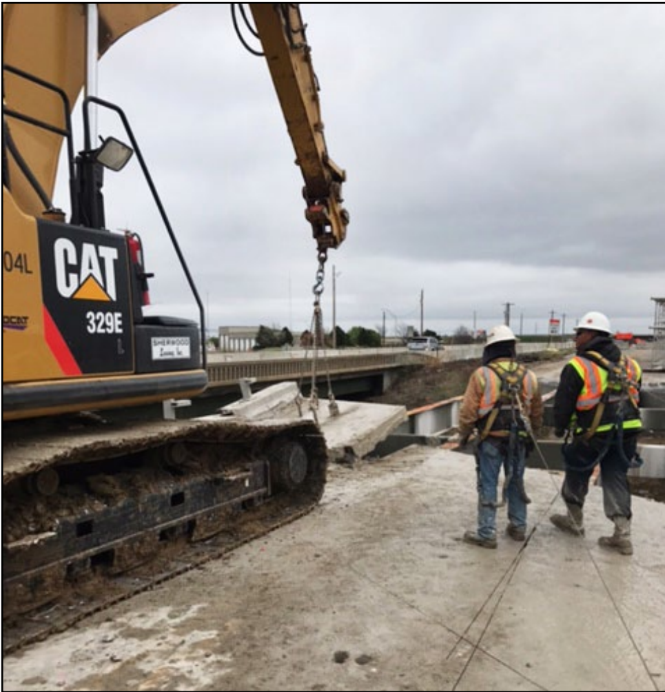
KTA crews remove the bridge deck of eastbound Kellogg bridge in Wichita, near 127th Street, that crosses over the Kansas Turnpike.
