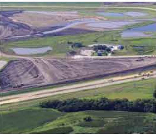
This photo shows the wetlands and the SLT under construction in April 2016.
