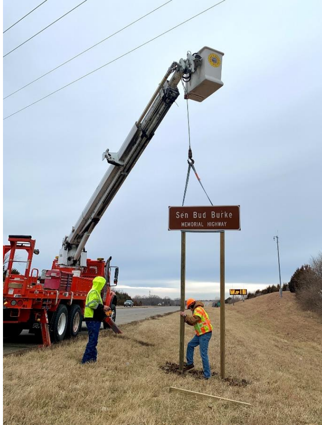
KDOT crew aligns signposts to set in steel sleeves preset underground. Photo by Delaney Tholen, KDOT.
