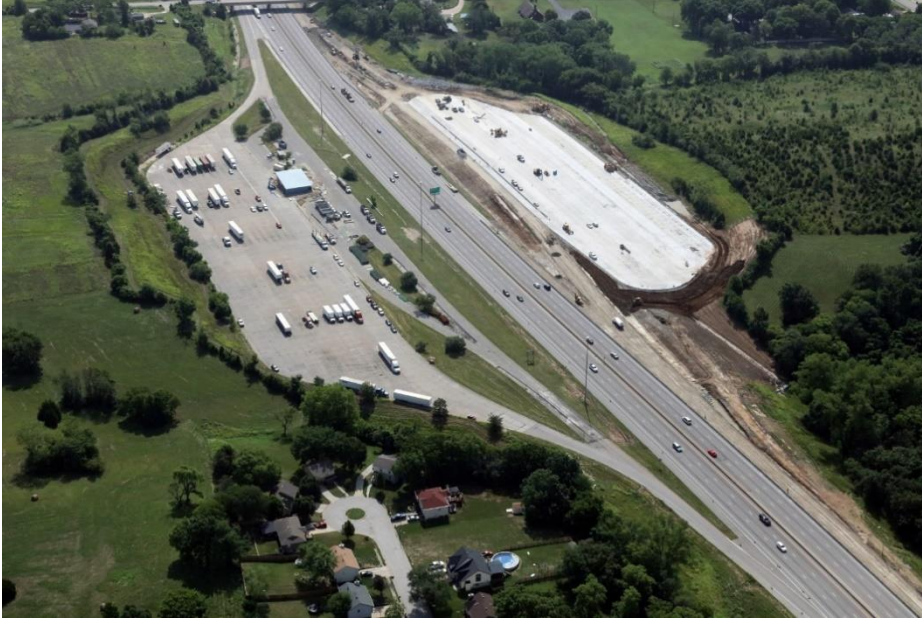
Truck staging area on I-70 at the Turner Diagonal in WYCO (July)
