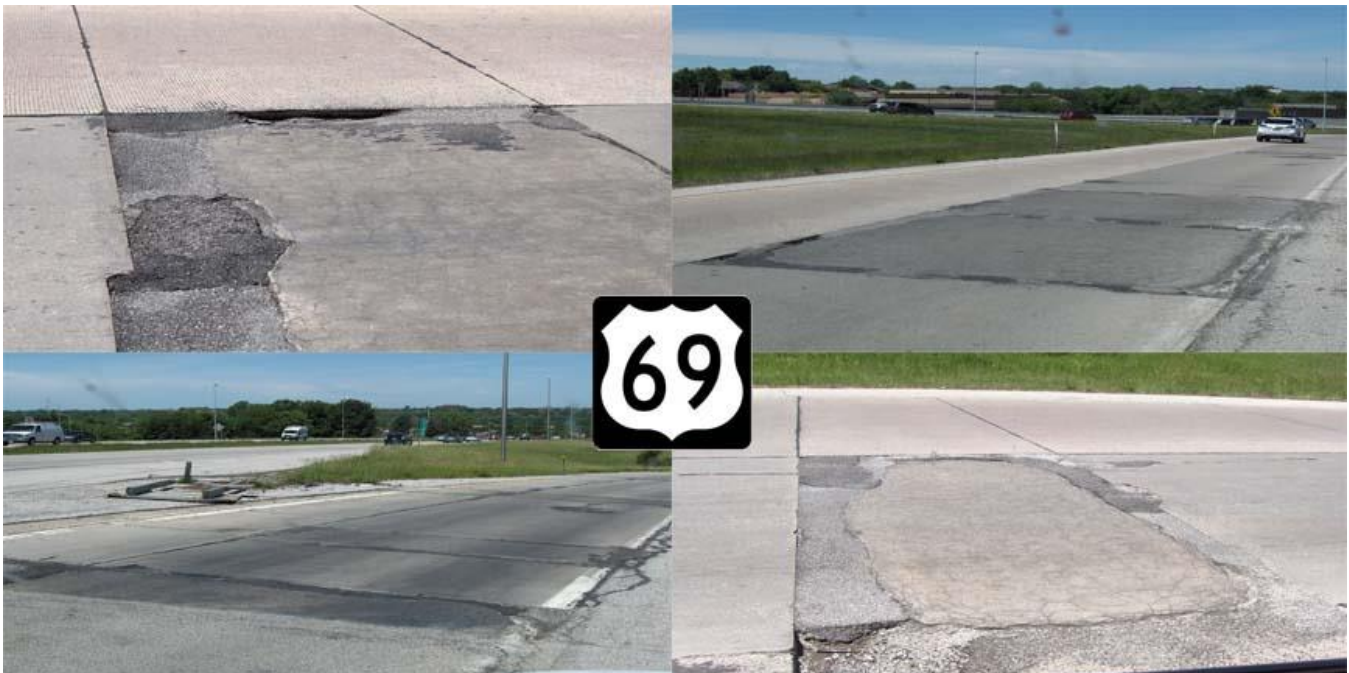
A look at the existing deteriorating pavement on the NB U.S. 69 Bridge over 119th Street.
