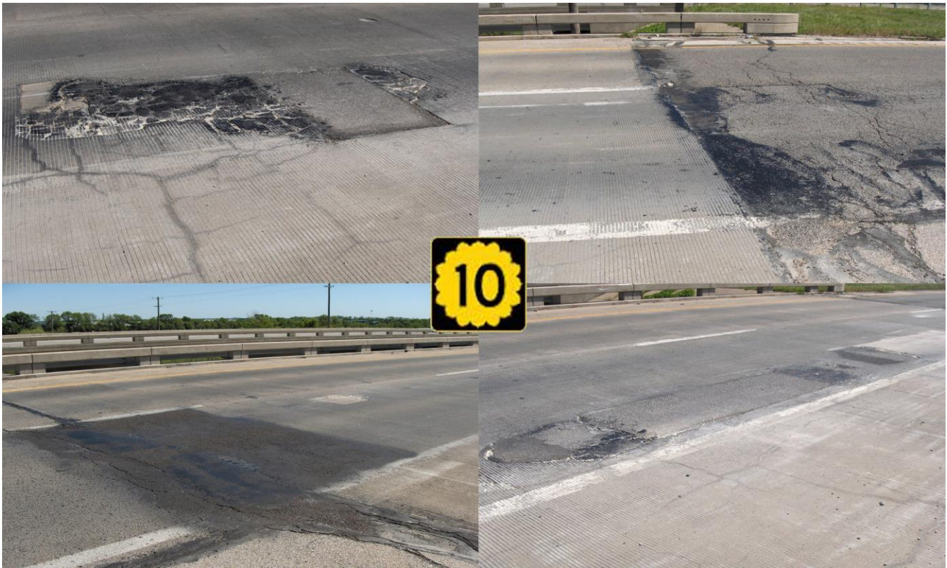
A 'before' look at the deteriorating pavement on the EB K-10 Bridge over Sunflower Road.
