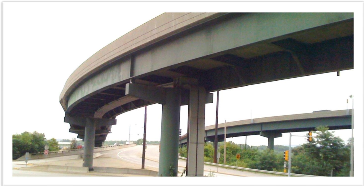
The girders and piers on this ramp structure in Wyandotte County are Fracture Critical Members.
