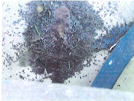
Photo 4: Guano deposits visible from bridge deck, on top of pier
