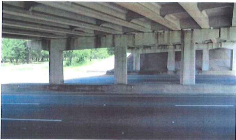
Photo 9: Staining on sides of pier caps
