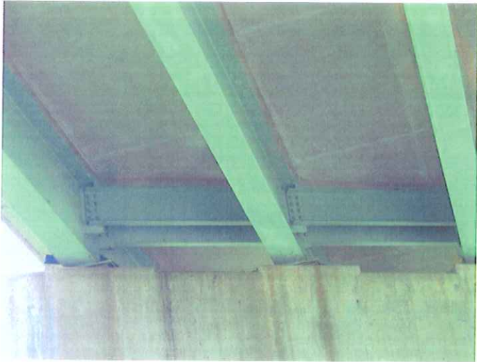
Photo 10: Guano staining on side of pier
