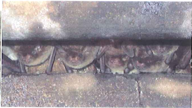
Photo 2: Visible bats within an expansion joint
