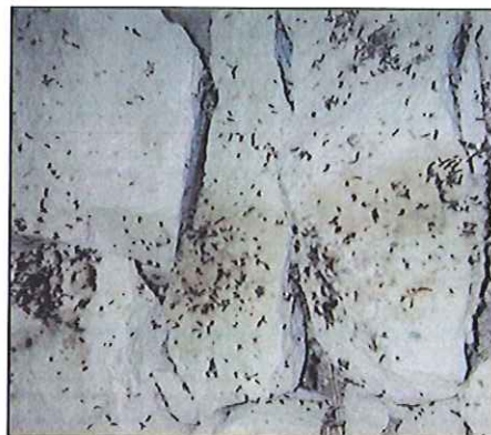
Photo 6: Bat Guano on Rip Rap
