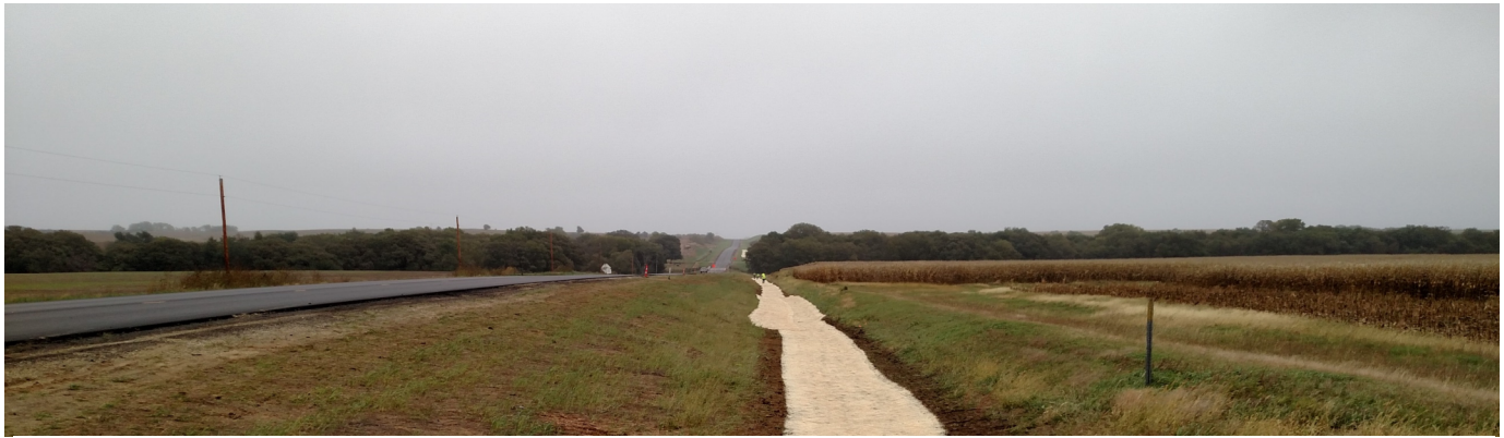
Stabilized area with Class II mat to protect the channel bottom from washing out
