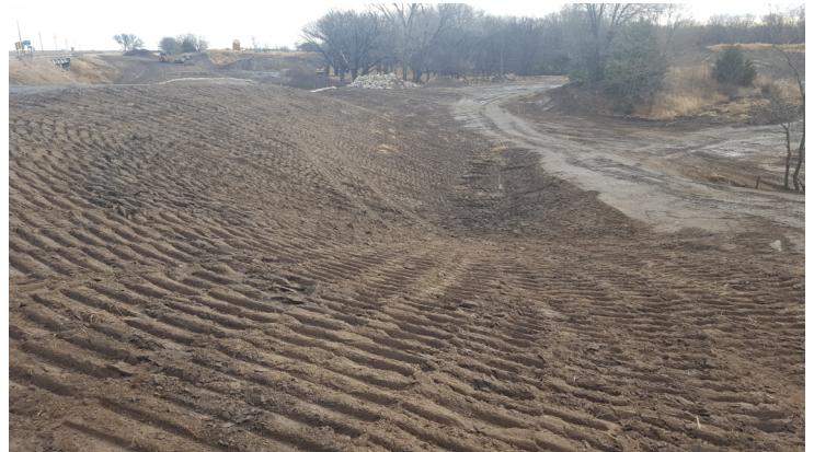
Cat tracking alone is not a sufficient bmp in soil stabilization. This area should be considered inactive on an oversight inspection.
