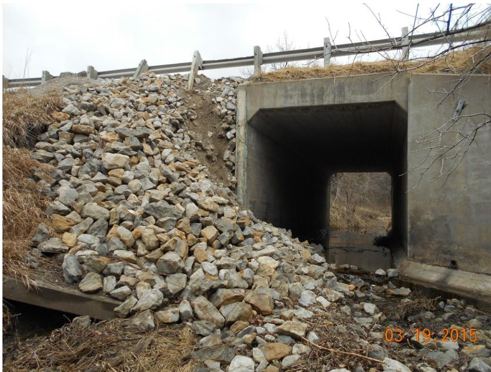
Photo above shows right wing wall in place, damaged left wing wall has been removed and replaced with crushed rock for now.
