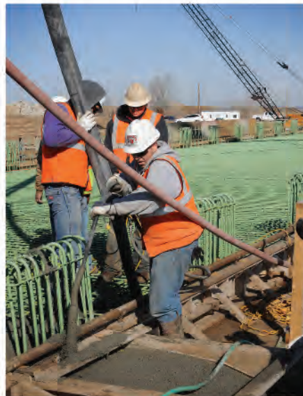
Concrete is poured on the deck of an I-70 bridge in Saline County.
