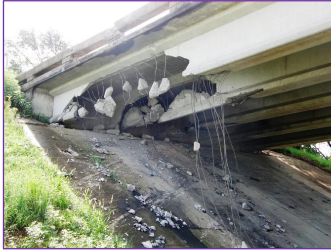
The Georgia Road bridge over U.S. 169 sustained damage in a vehicle crash. (KDOT photo)
