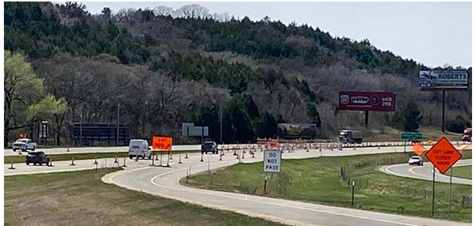
Westbound traffic is reduced to one lane at the entrance of the work zone for the I-70 pavement replacement project at Junction City. Photo by Ashley Perez
