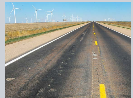
Mill and overlay work started early on a stretch of U.S. 50. Photo by Multimedia Services
